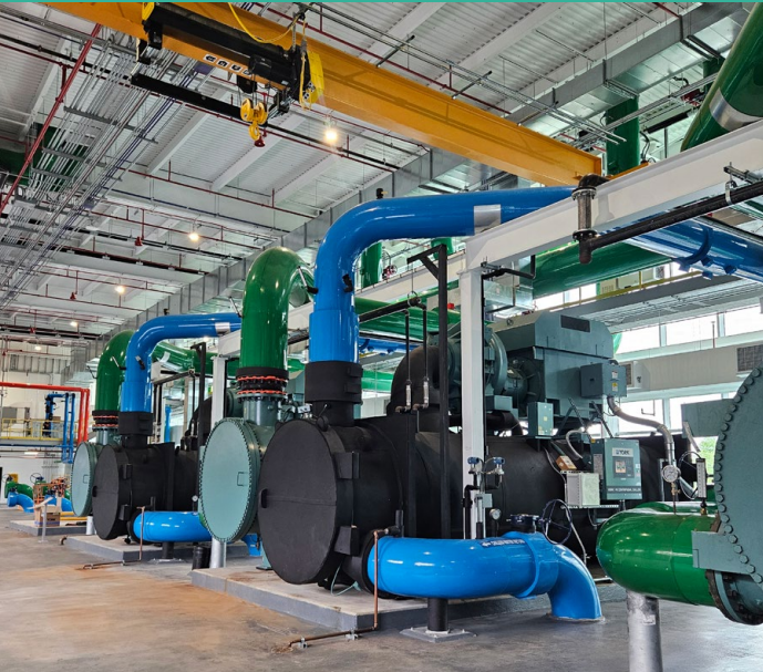
University of Pittsburgh Central Utility Building
